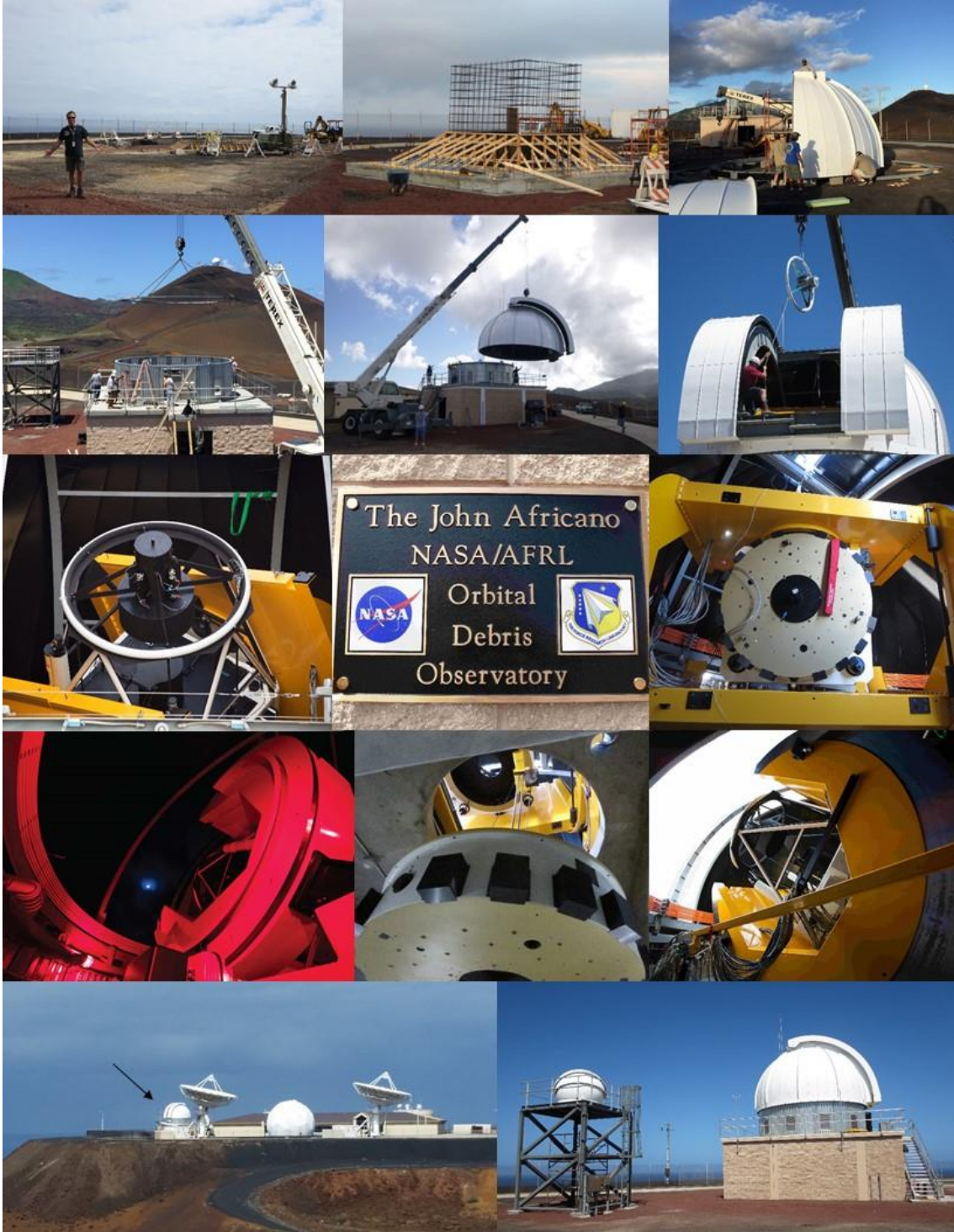
Fig. 4. Construction of MCAT on Ascension Island. Photo credit for the three full telescope images, Ben Hanna, Royal Air Force.
