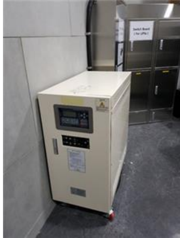
Fig. 1. Frequency converter and UPS
