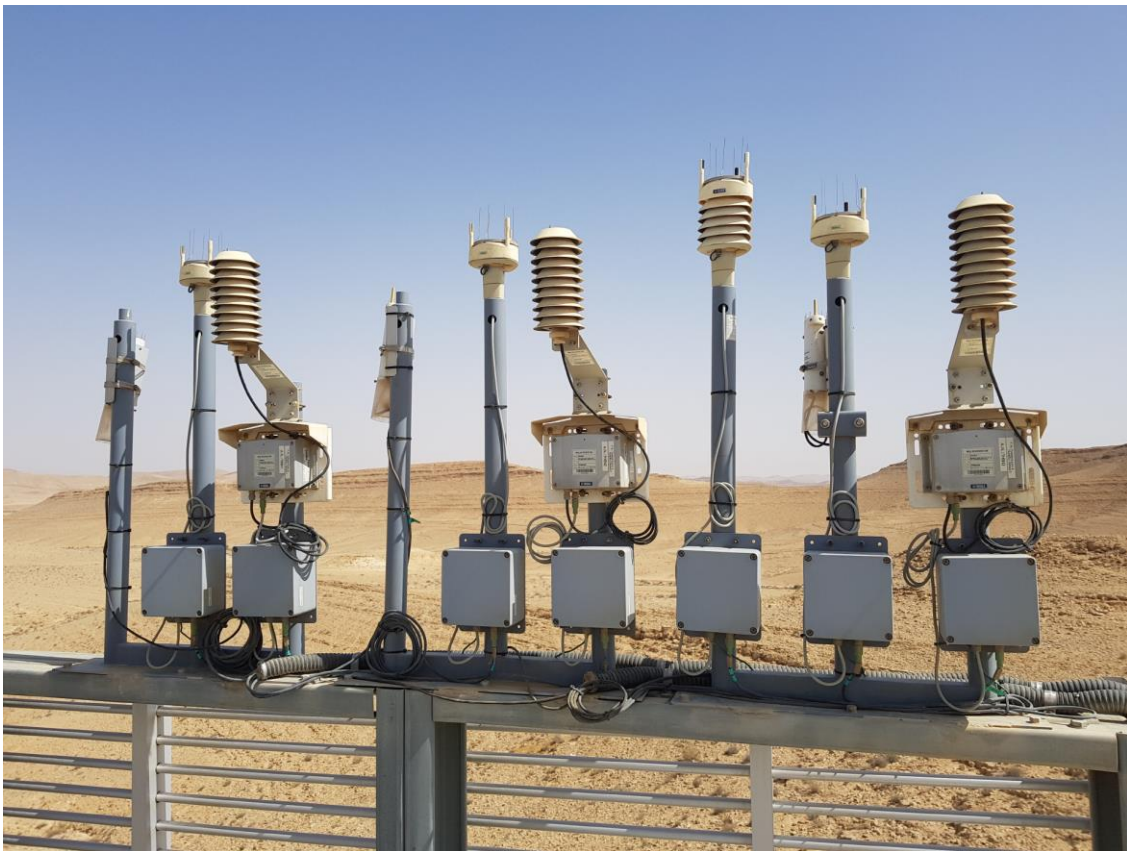
Fig. 3. Multiple weather sensors for each key weather device at OWL station
